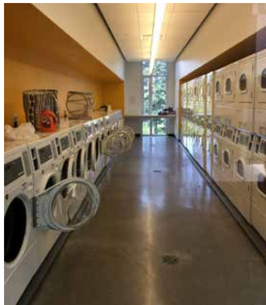
Residential laundry facilities.
