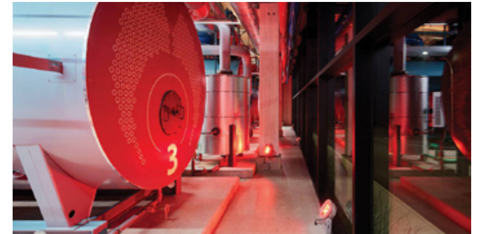
Photo: District Energy Plant - UVic Photo Services
