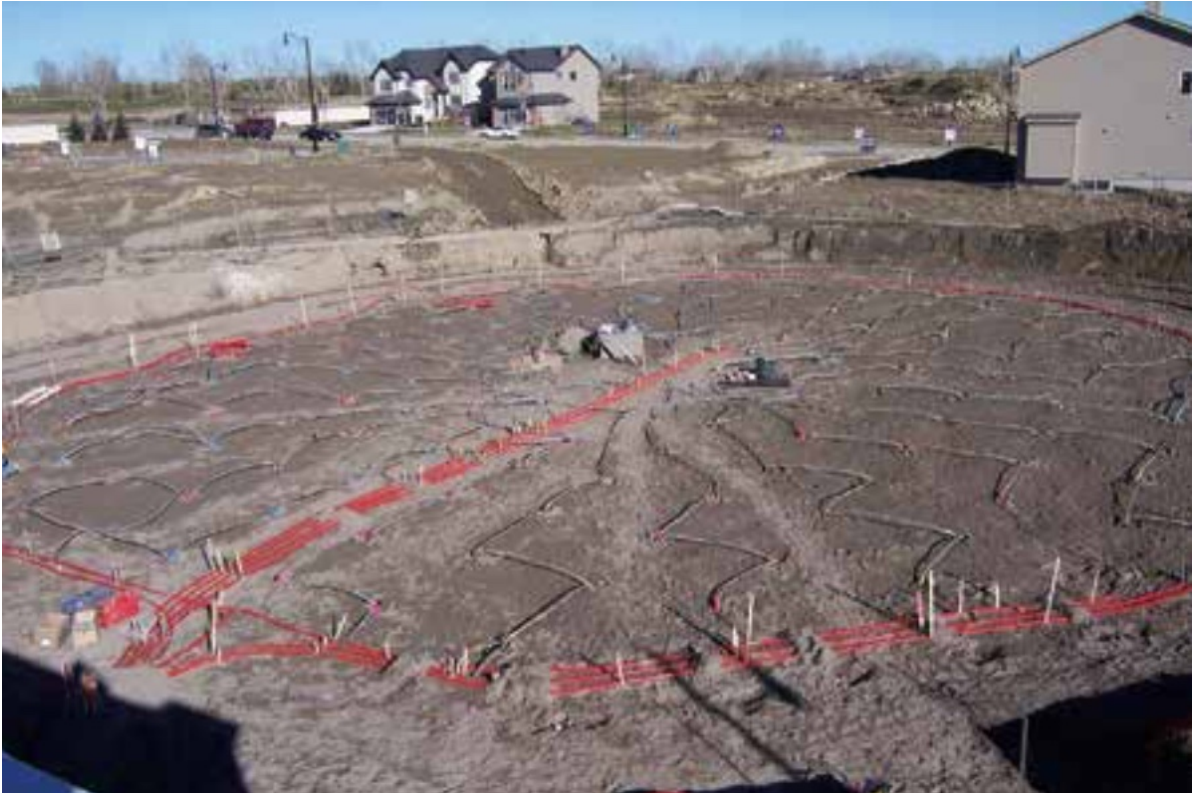
Figure 4: A view of the BTES field in the Alberta solar thermal storage project [21]
