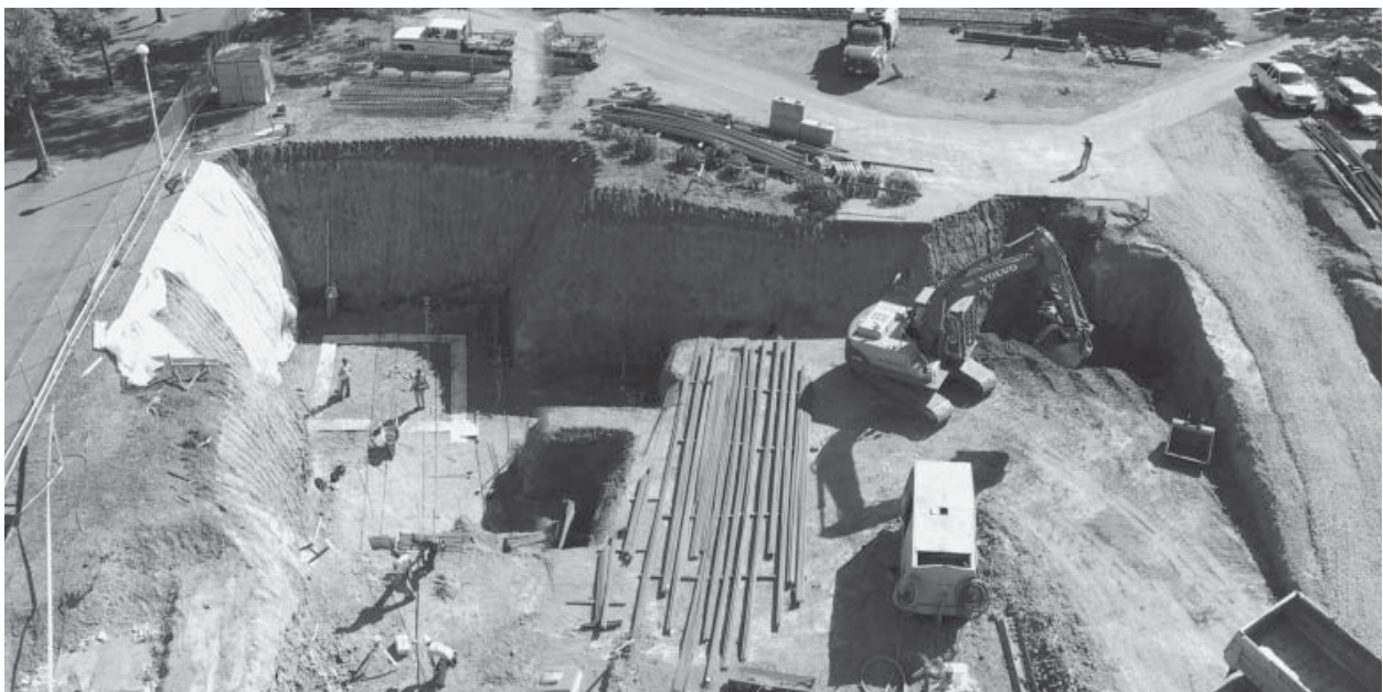
Top left: dump trucks are loaded during site excavation. Top right: cement and steel girders form the beginning of the foundation. Bottom: the view of the construction site from the roof of the McPherson Building. (Photos by Kate Daley, University Librarian's Office; Wendie McHenry, University Librarian's Office; and Don Lovell, Facilities Management, respectively.)
